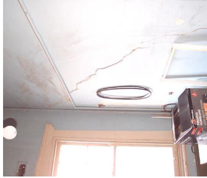
Cracking, south wall
