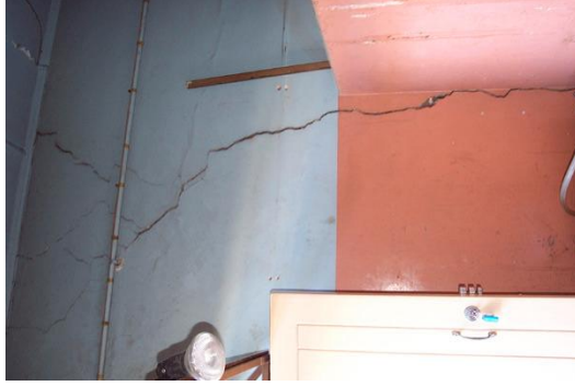
Structural crack – south wall (north same)
