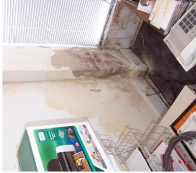
Penetrating damp – south-east cnr
