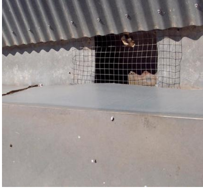
Typical sump box in box gutter – depth as little as 70mm in places
