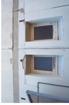
Failed render over toilet windows
