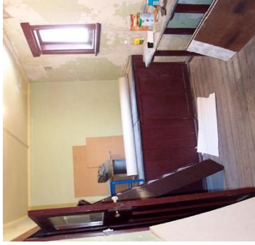
West store room – damp affected wall
